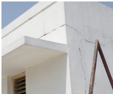
Cracks in Guria School walls
